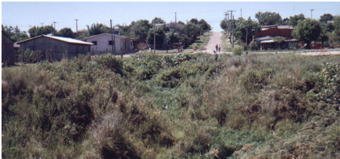
Picture 04: Water flowing of the street direct throwing at the streams have increase the erosion.
