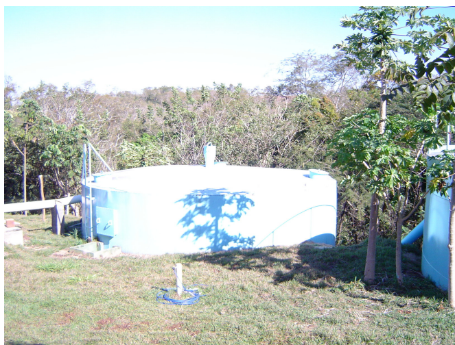
Partial vision of the Station of Treatment of Effluent
