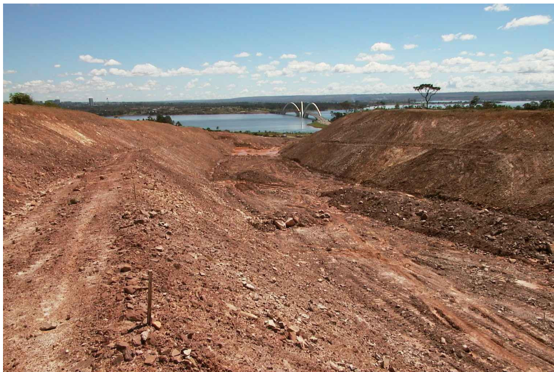
Figure 2 - Sight of cut slopes in highway EPDB/EPCT after concluded the excavating services.
