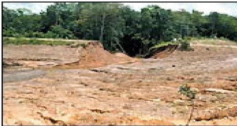
Picture 02 - Destroyed dam near the area of the collapse.
