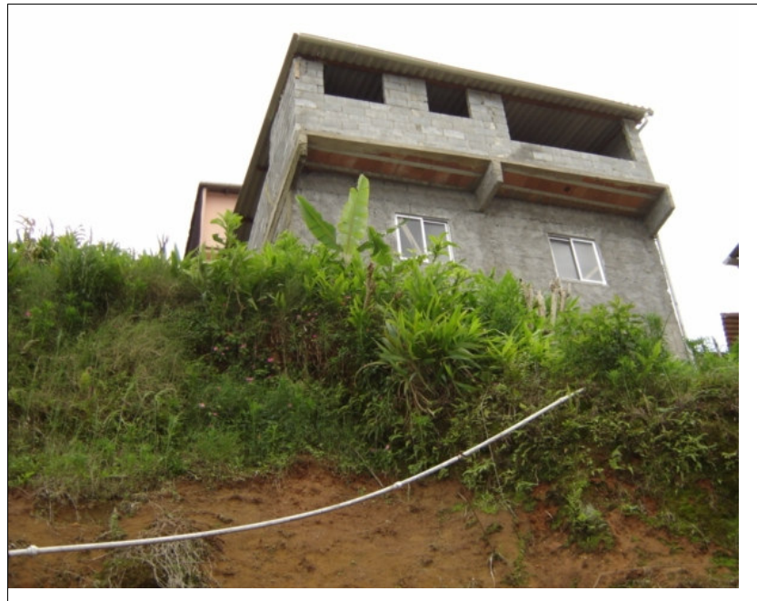
Figure 4: House built on a very unstable slope with slope angle over 70°, with a cut on the talus, characterizing a level 5 risk on the Table of Vulnerability Factors (Valparaiso, 2004).
