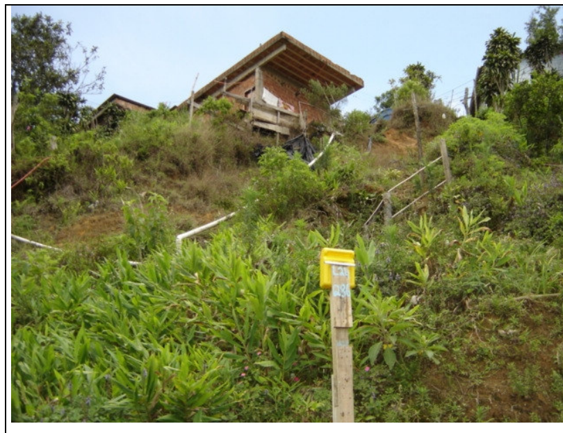
Figure 6: House with deficient structure, soil sinking and the presence of clandestine pipes with water leakage, outlining level 5 risk on the Table of Landslide Vulnerability (Valparaiso, 2004).
