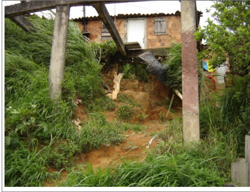
Figure 5: House with deficient structure, presence of cracks and soil sinking, outlining level 5 risk on the Table of Landslides Vulnerability Risk (Valparaiso, 2004).
