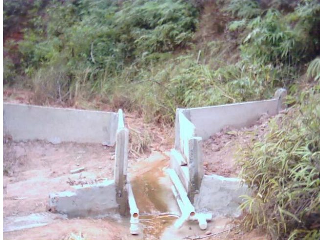
Fig. 3 – This picture shows an embankment with a floodgate that was installed into the gully channel for collecting data about sediments transported at the bottom (ROCHA, Erica – 2004)
