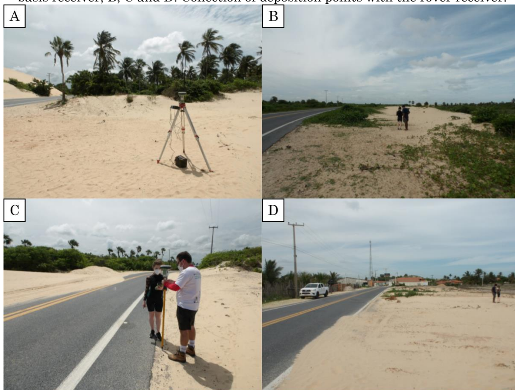
Figure 3 – Collecting control coordinates of sediment disposal area points. A. Geodetic GPS basis receiver; B, C and D. Collection of deposition points with the rover receiver.
