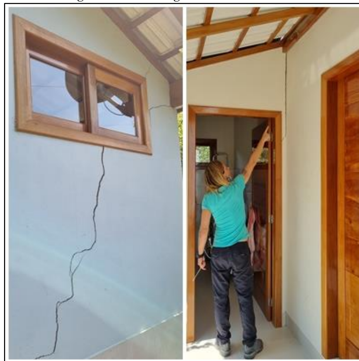
Figure 13 - Damage to the residence
