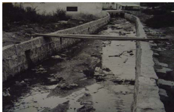
Fig. 3b - Excerpt from the work of canalization of the river Criciúma in granite stone, 1980s.
