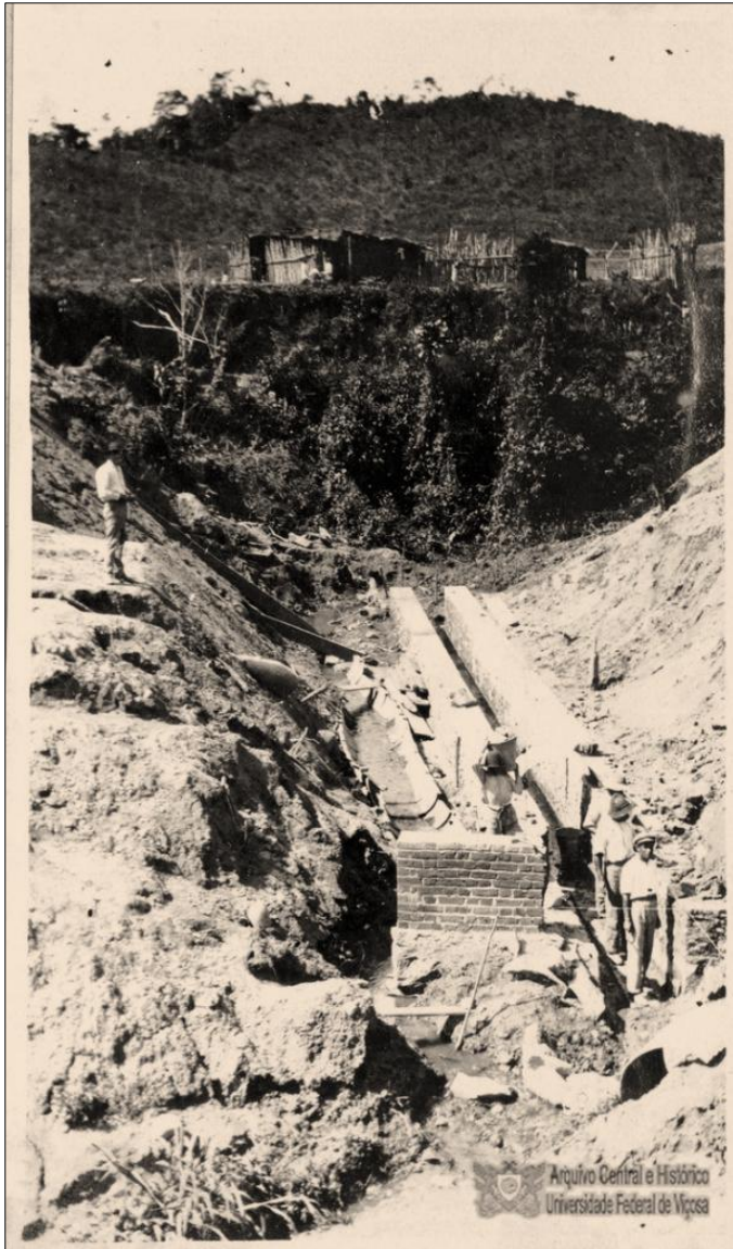
Figure 3 – Córrego dos Barbados Drain, ([undated]). Workers constructing the drain in a section that cuts through one of the ESAV roads
