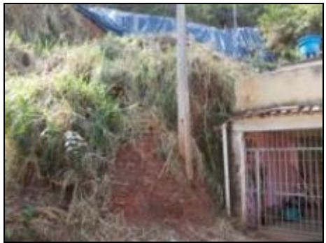
Point 53 - Street at the top of the slope without paving and drainage
