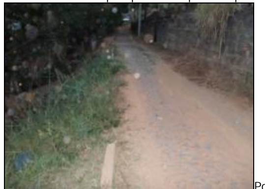
Point 15 - Damaged drainage at the top of a slope
