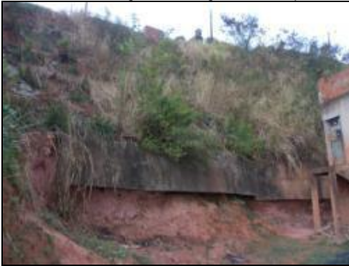
Point 18 - Undermining of contention wall
