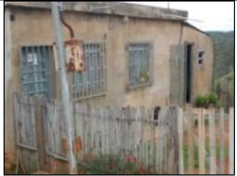
Point 49 - Cracks in home built on a landfill
