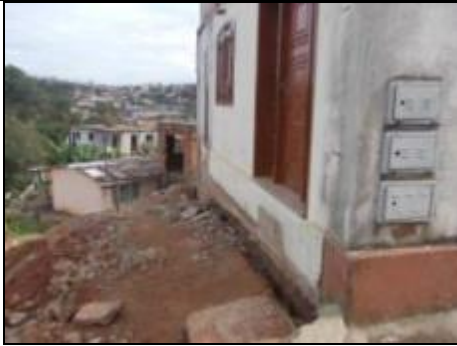
Point 03 – Sliding on top of a slope
