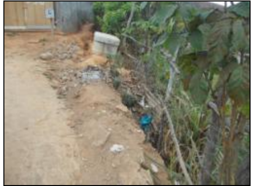
Point 17 - Dump disposal on top of a slope
